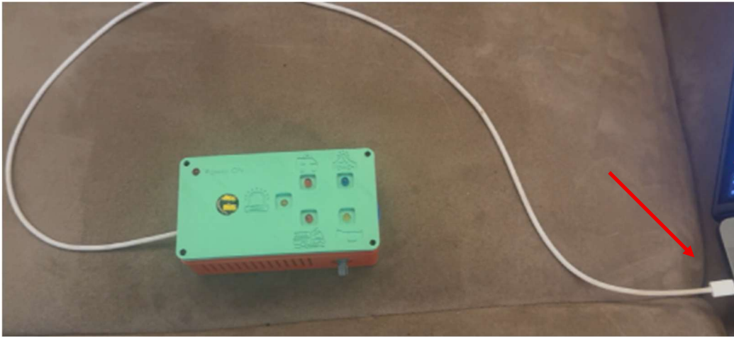
Figure 15. UBS connection to power on.
